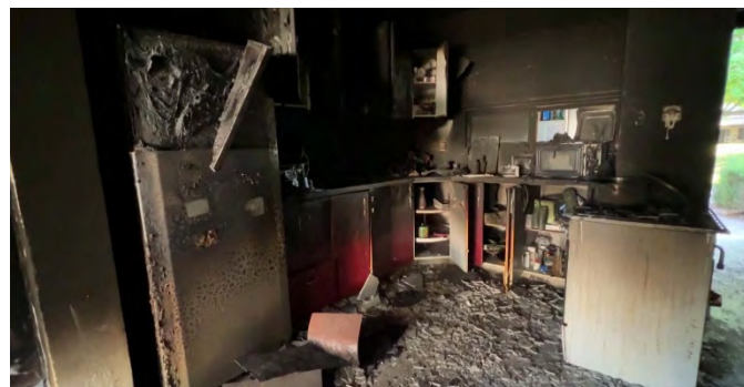
Damage to a house in Kibbutz Holit from fire Source: KAN 7.10.23 Digital Memorial Project
