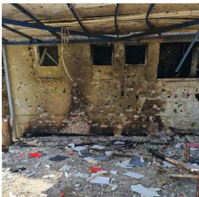
Damage to a home in Kibbutz Be'eri. Source: KAN 7.10.23 Digital Memorial Project
