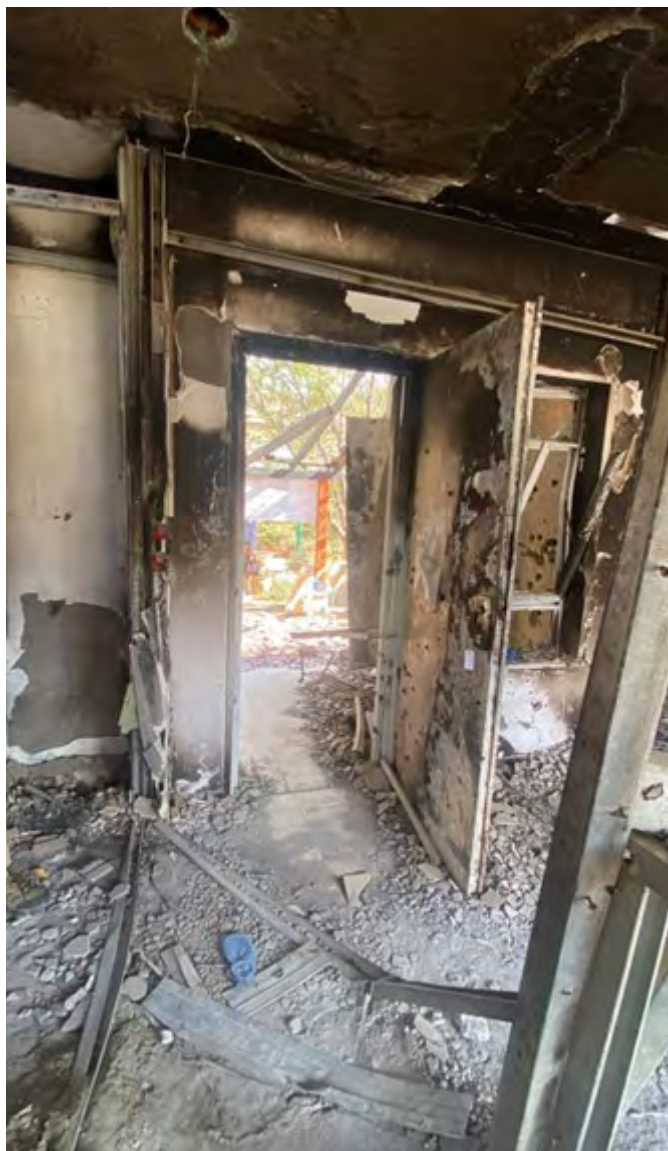
Damage to a home in Kibbutz Be'eri. Source: Photo taken on Lord Roberts' visit to the Kibbutz in August 2024
